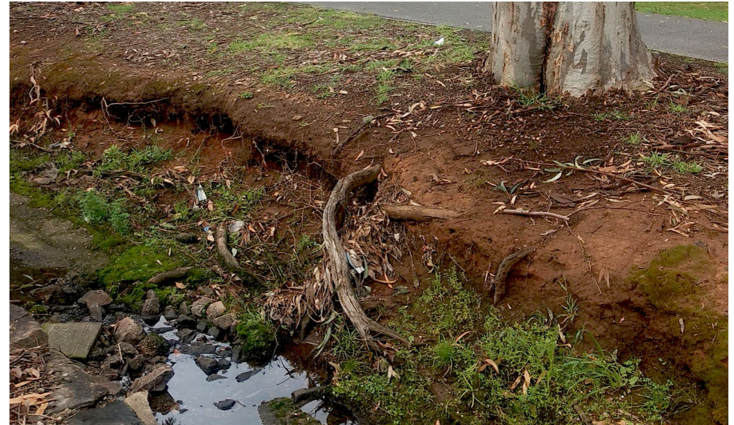
Exposed tree roots within drainage channel
