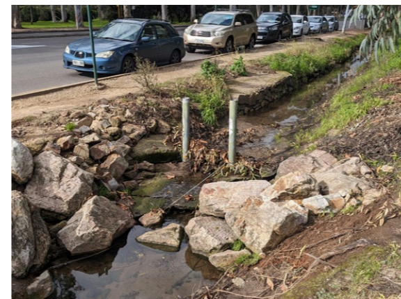
Existing drainage channel in degraded condition
